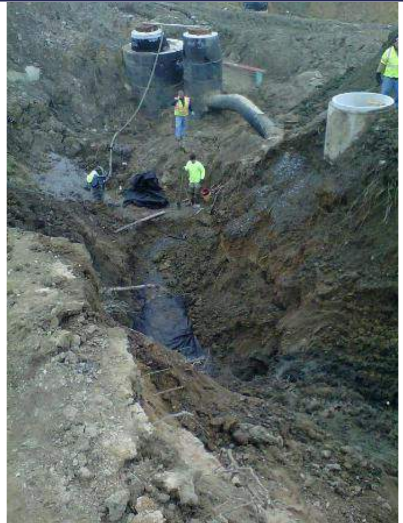
View: Underdrain for Cutoff Wall
