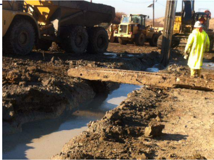
View: Upgradient Cutoff Wall
