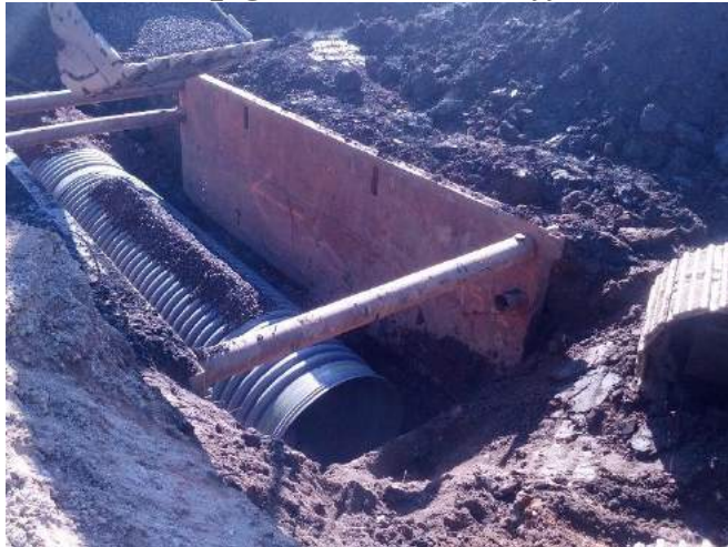
View: Upgradient Stormwater Pipe
